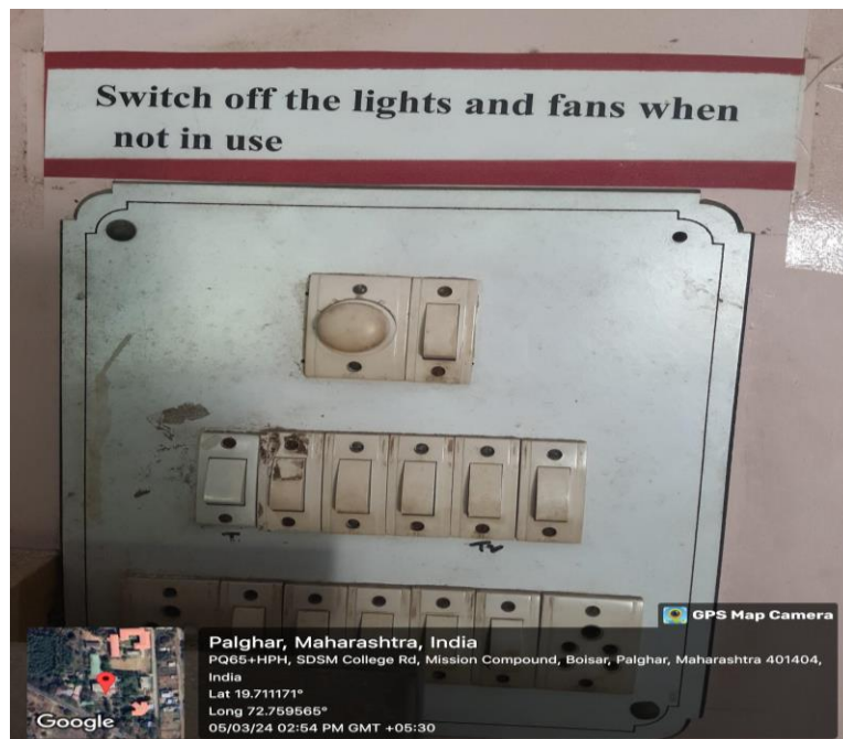
Switch Boards Label with energy saving Instructions like "SWITCH OFF and ON" at Biotechnology Laboratory
